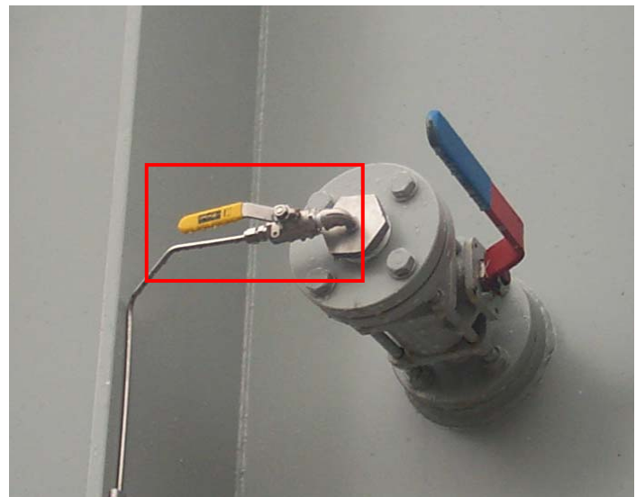
Figure 2: Oil shut off valve
