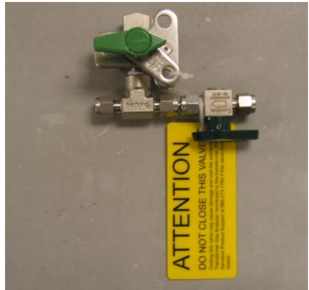
Figure 3: DGA sample port
